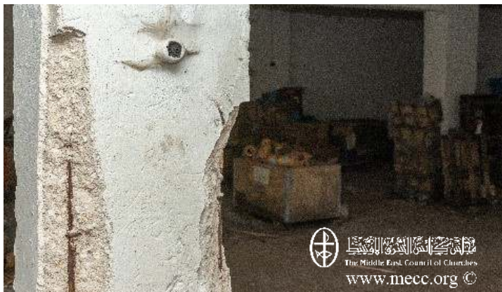
The basement of the building in Midan needs reinforcement to ensure safety to all residents
